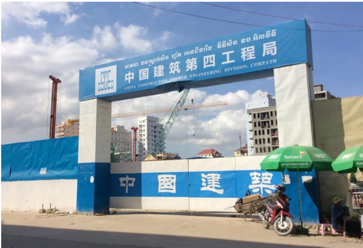
Chinese real estate construction contracted to CSCEC, Phnom Penh, Cambodia (By Inclusive Development International)
